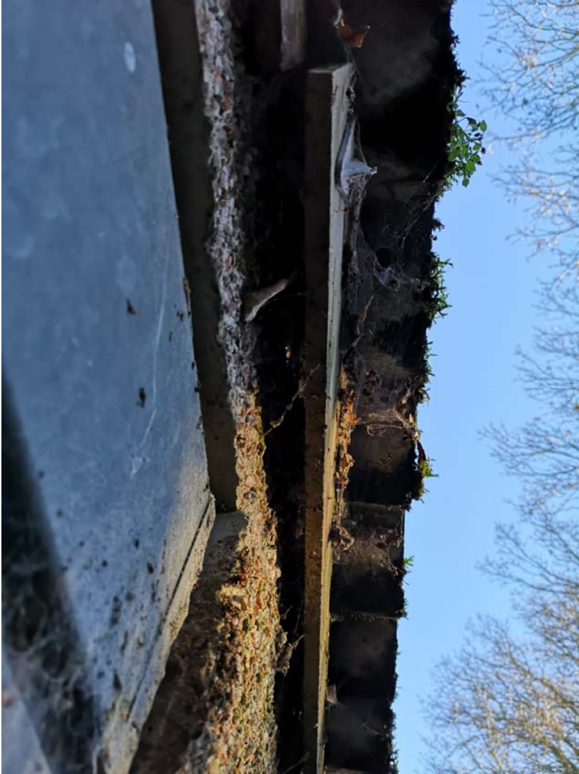
Photograph 7.7.4: Stakes Lane garages – under barge boards, 16/01/2019, standard lens
